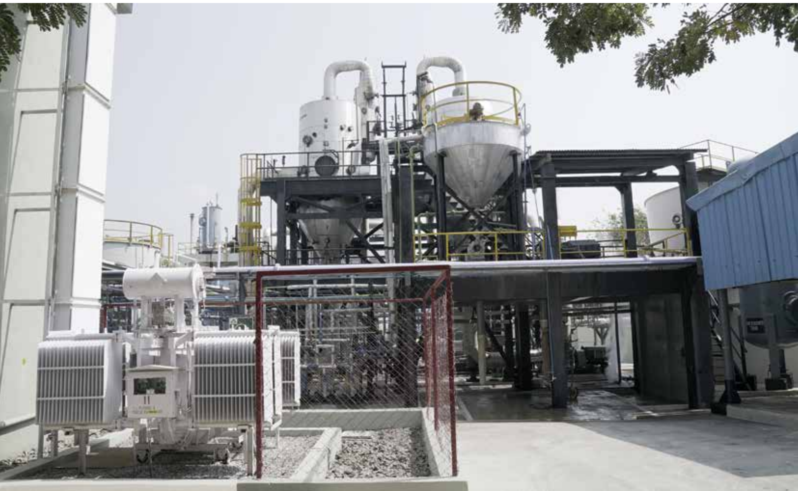
Zero Liquid Discharge (ZLD) facility, Chemplast Sanmar, Mettur.
